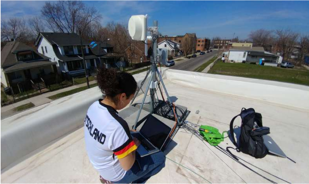
Fig. 3 - Digital Steward assembling and checking a MESH antenna – © Detroit Community Technology Project – Allied Media Project – https://detroitcommunitytech.org/
