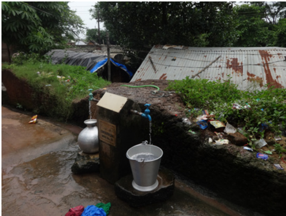
Fig. 10 – Drinking water facilities, Mahishakhala
